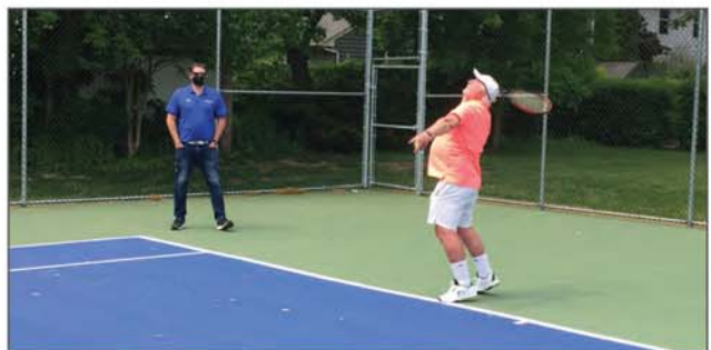
Parks and recreation manager Kevin Turcotte and NOTL Tennis Club president Hugh Dow check out the new courts at Memorial Park, which will be used for the Canada Summer Games. The older courts will be resurfaced in time for the August competition, and painted blue to match the new courts. (Mike Balsom)
